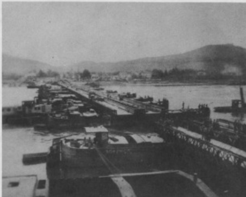
Fig. 41. LAST FLOATING BAY BEING JOINED TO BRIDGE. TUGS HAVE NOT BEEN CUT LOOSE.
