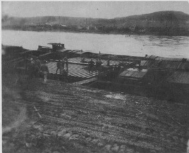
Fig. 21. LANDING BAY PIER AND END FLOATING BAY PIER READY FOR INSTALLATION OF END FLOATING BAY
