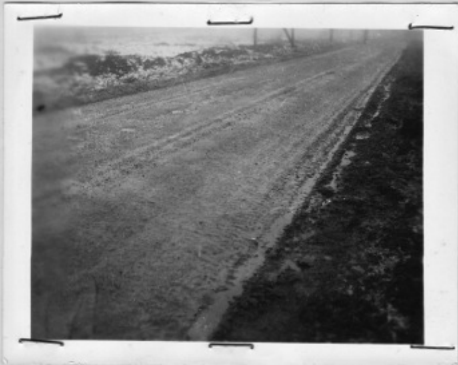
N-51 EUPEN TO MONSCHAU ROAD BEFORE FAILURE
