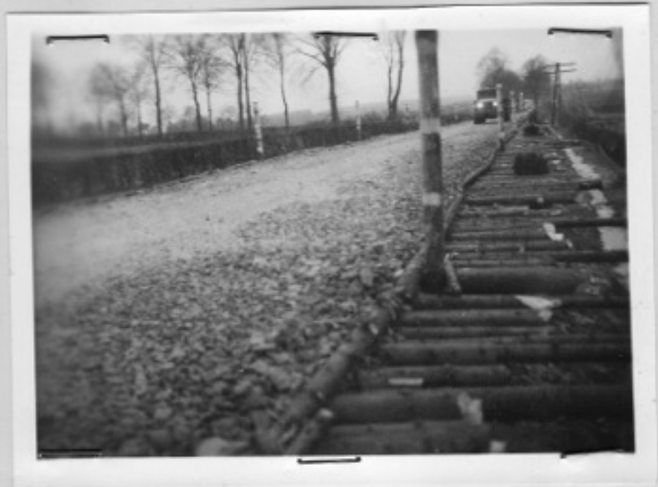
N-31 EUPEN TO MONSCHAU CORDUROY, COMPLETE AND READY FOR TRAFFIC, 207 ENGINEER COMBAT BATTALION
