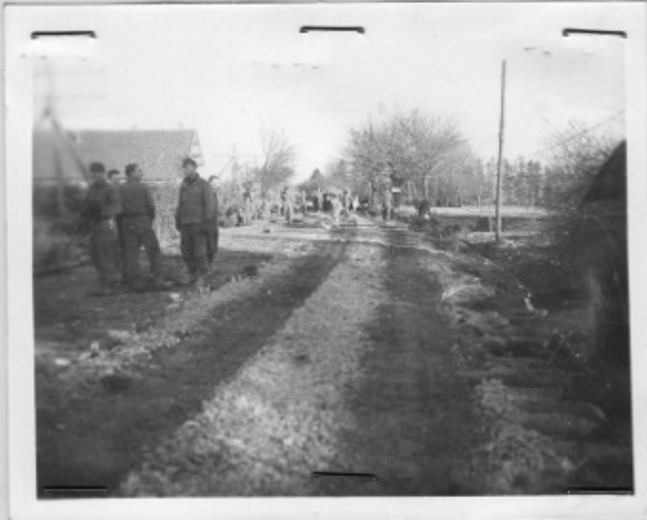
N-31 EUPEN TO MONSCHAU CORDUROY: ONE LANE COMPLETE; SECOND LANE UNDER CONSTRUCTION BY 207TH ENGR C BN
