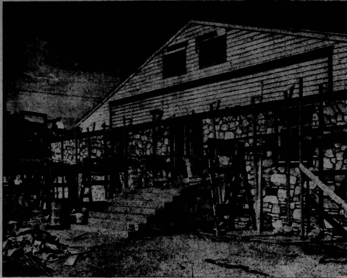
FRONT VIEW of the new NCO Club Building located on the southeast corner of the parade ground beside the Fire Station. Construction on the club is practically completed, and formal dedication ceremonies will be held on Organization Day, 22 November.
