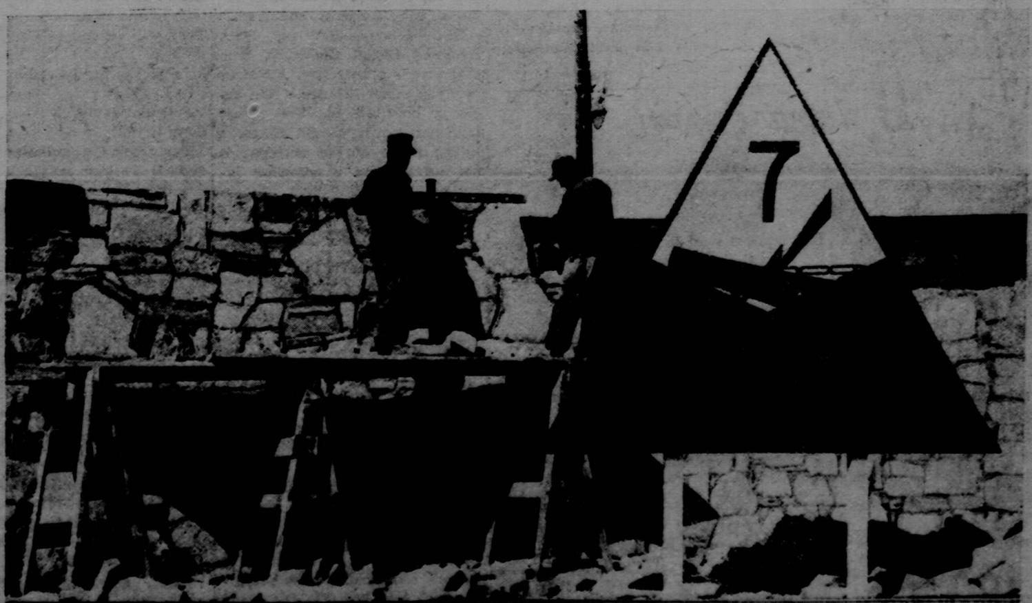
A MONUMENT dedicated to the memory of Corporal Harold W. Roberts, World War I hero and the man for whom Camp Roberts is named, is nearing completion. PFC Joe S. Lewis and Sgt. Felix Kozel, both of the 107th Replacement Company, are shown here laying the flagstones. The monument will be located in a small square near the main gate. On one
