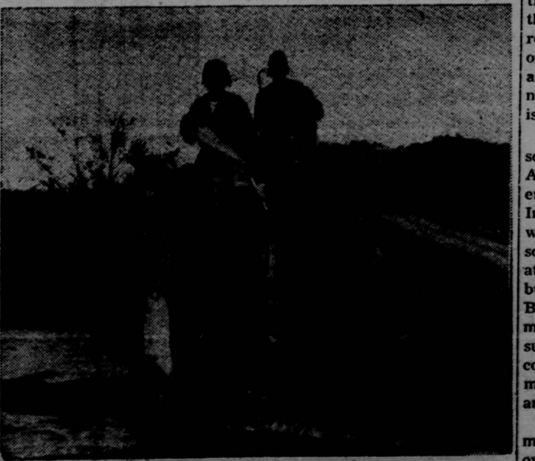
TAKING A BREAK during final construction of a 215-foot bridge spanning the Nacimiento River at Camp Roberts are those men of Company B, 23rd Armored Infantry Battalion, 7th Armored Division. From left to right, bottom to top, are Privates Eugene Palermo, Amillio Montes, 1st Lieutenant Alfred H. McCluskey, Private James B. Evanston and Private First Class Joseph Sealler. (Camp Roberts PIO Photo).
